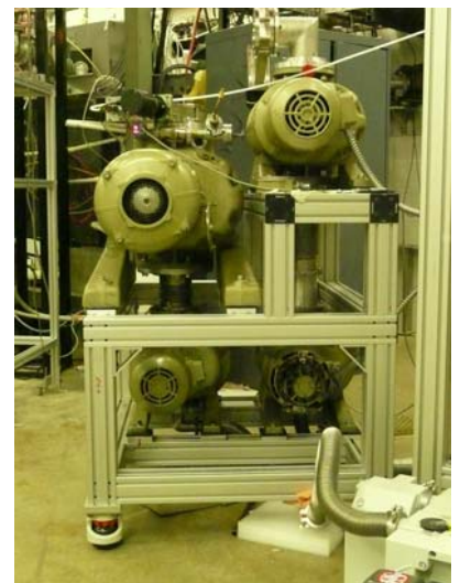
The Roots Blowers pumps have a total weight of 2000 lbs. Mounted on their own stand they can be moved easily.
