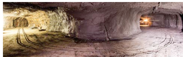
Figure 5: This cavern will house the CASPAR experiment. The left side has had shotcrete applied and will soon cover the ribs on the right.
