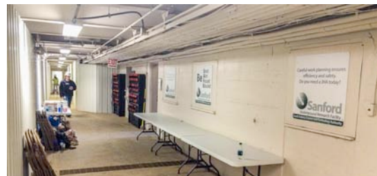
Figure 9: Junior Facility Engineer Andrew Brosnahan inspects work at the Yates Ramp, which includes new signs with safety messages
